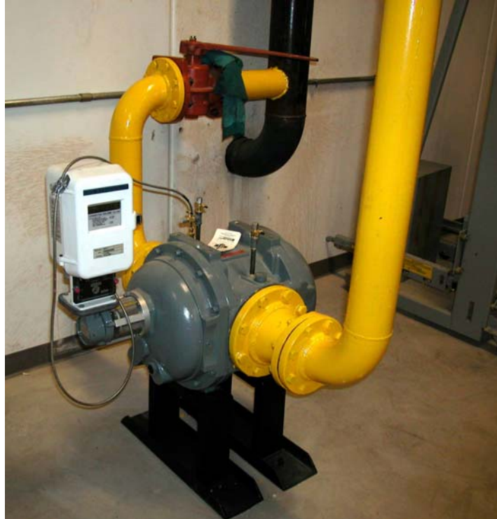
Figure 12: Natural Gas Sub-meter Installed for Data Acquisition Effort
